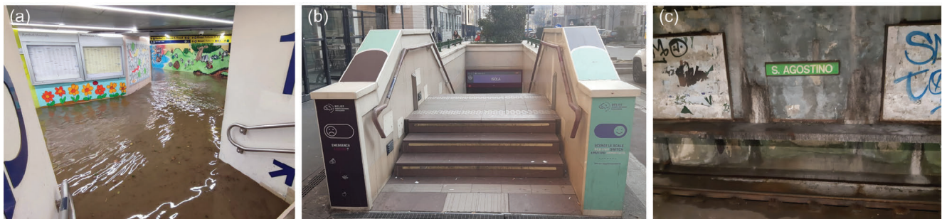
Fig. 4 - a) water and sediments inrush caused by the stormwater event of 31 st October 2023 at Garibaldi subway station; b) mitigation measures to floods at Isola station; c) corrosion of foundations at Sant'Agostino station (subway line M2) caused by groundwater/underground infrastructures interactions. All images have been taken by the authors.
