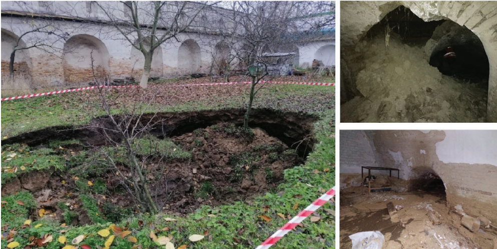
Fig. 5 - Photographs of sinkholes in the territory of the Metropolitan's Garden and the soil suffusion in the Metropolitan's Wine Cellar caused by the accident in October 2022.
