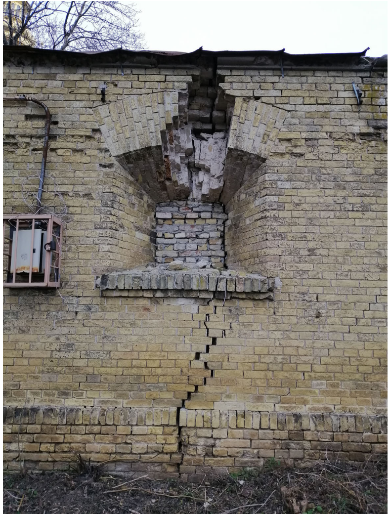
Fig. S11 - Crack in the defensive wall of Lavra (photo was taken in March 2024).
