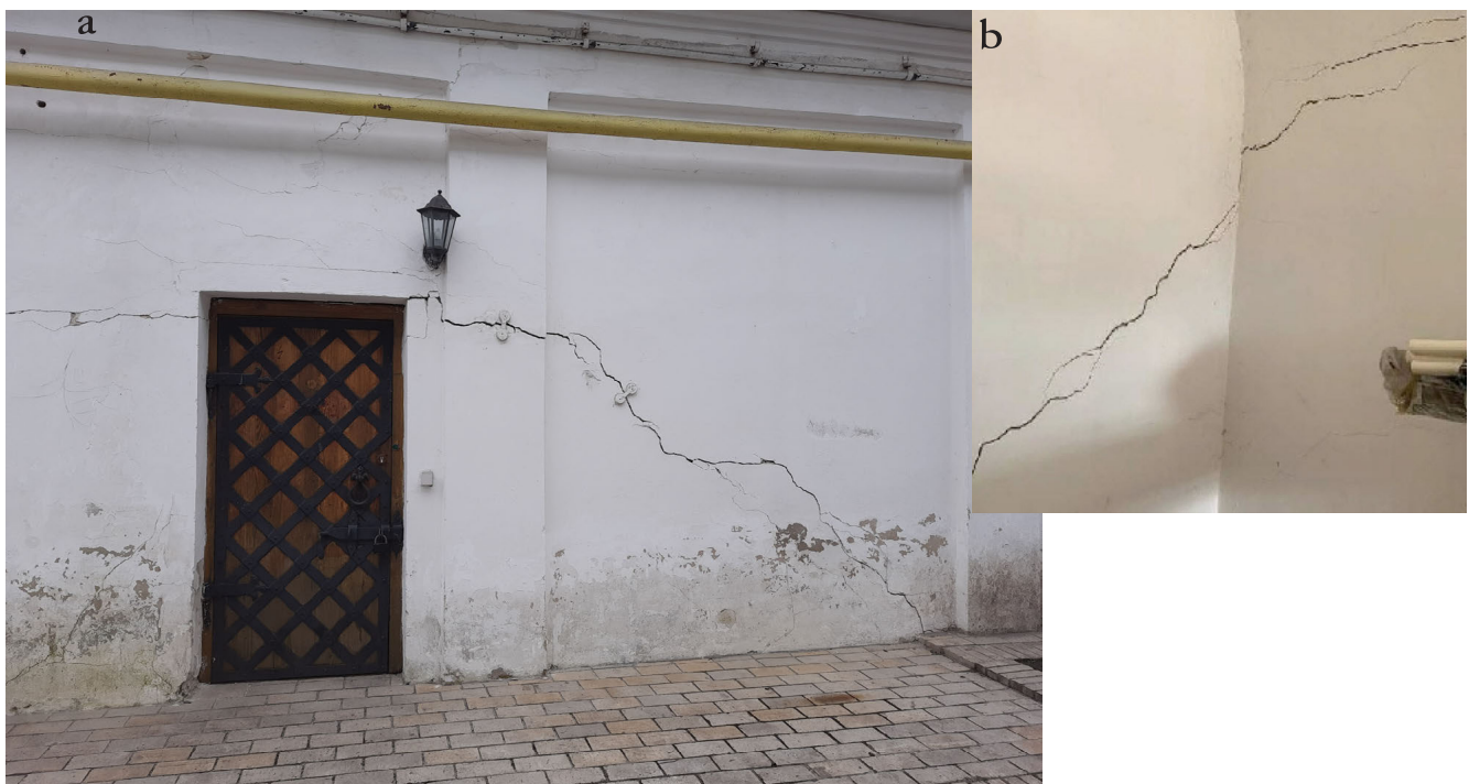
Fig. S10 - Cracks on the facade (a) and in interior premises (b) of Building no.21 caused by uneven subsidence of foundations (photo was taken on October 2021).
